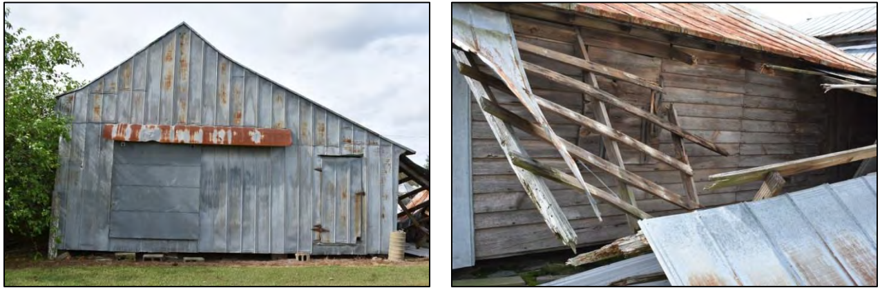
Figure 68: Left, east elevation with later sliding door and door to shed room; right, north elevation of shed
