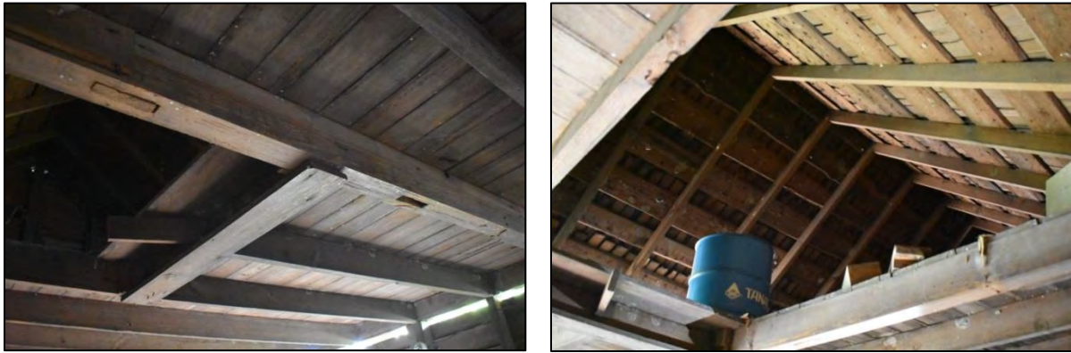
Figure 72: Left, view of building’s interior framing with ghost mortises of original partition wall; right, view looking up into loft, with common rafters and undersides of shingles visible
