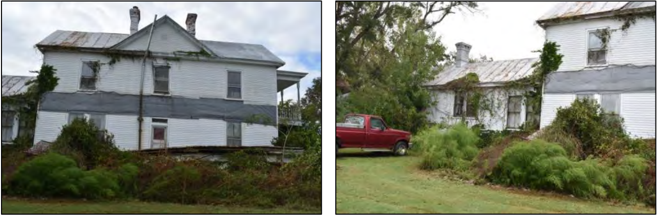
Figure 42: Left, north elevation with porch fallen away; right, north elevation detail with kitchen ell to rear— windows at center of image mark location of once-open breezeway
