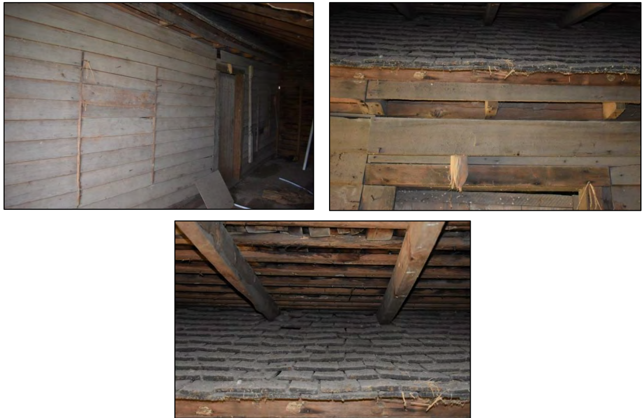
Figure 69: Left, view of house's original eastern exterior wall (now enclosed by shed roof addition); right and bottom, view of original wood shingle roof (now covered by roof of addition)
